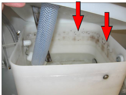
Figure 16.5g: Reservoir lid removed showing mold growth.
