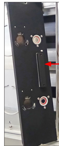
Figure 10.1b: Interior of black panel showing uninsulated temperature sensor.
